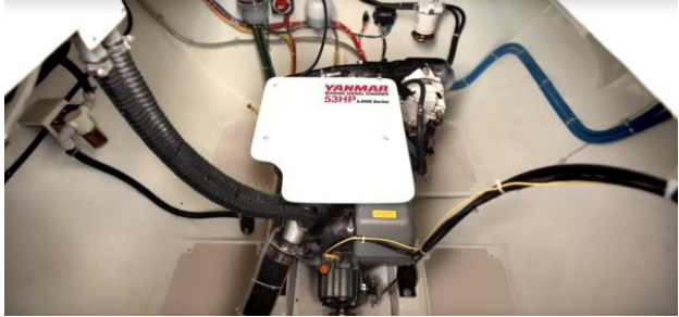
Very large engine room
